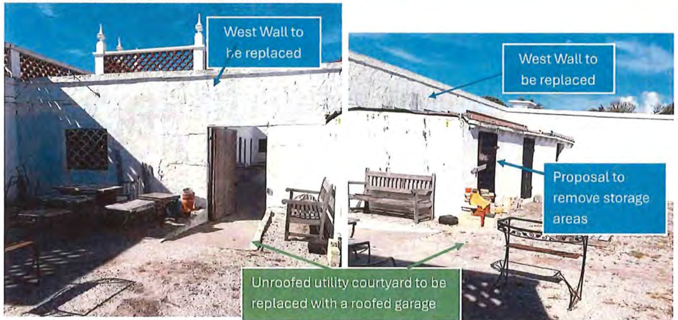
Interior of the west wall facing the unroofed utility courtyard. For the new garage the existing wall will be replaced with new and in addition a parapet wall will be installed on top of the wall.
